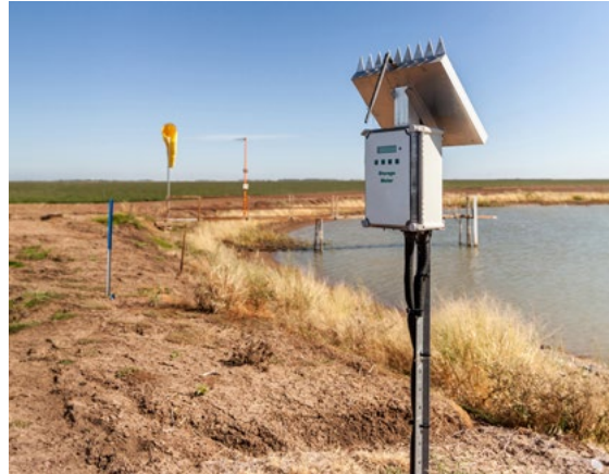
Water meter for accurately measuring water take. Photo: NRAR
